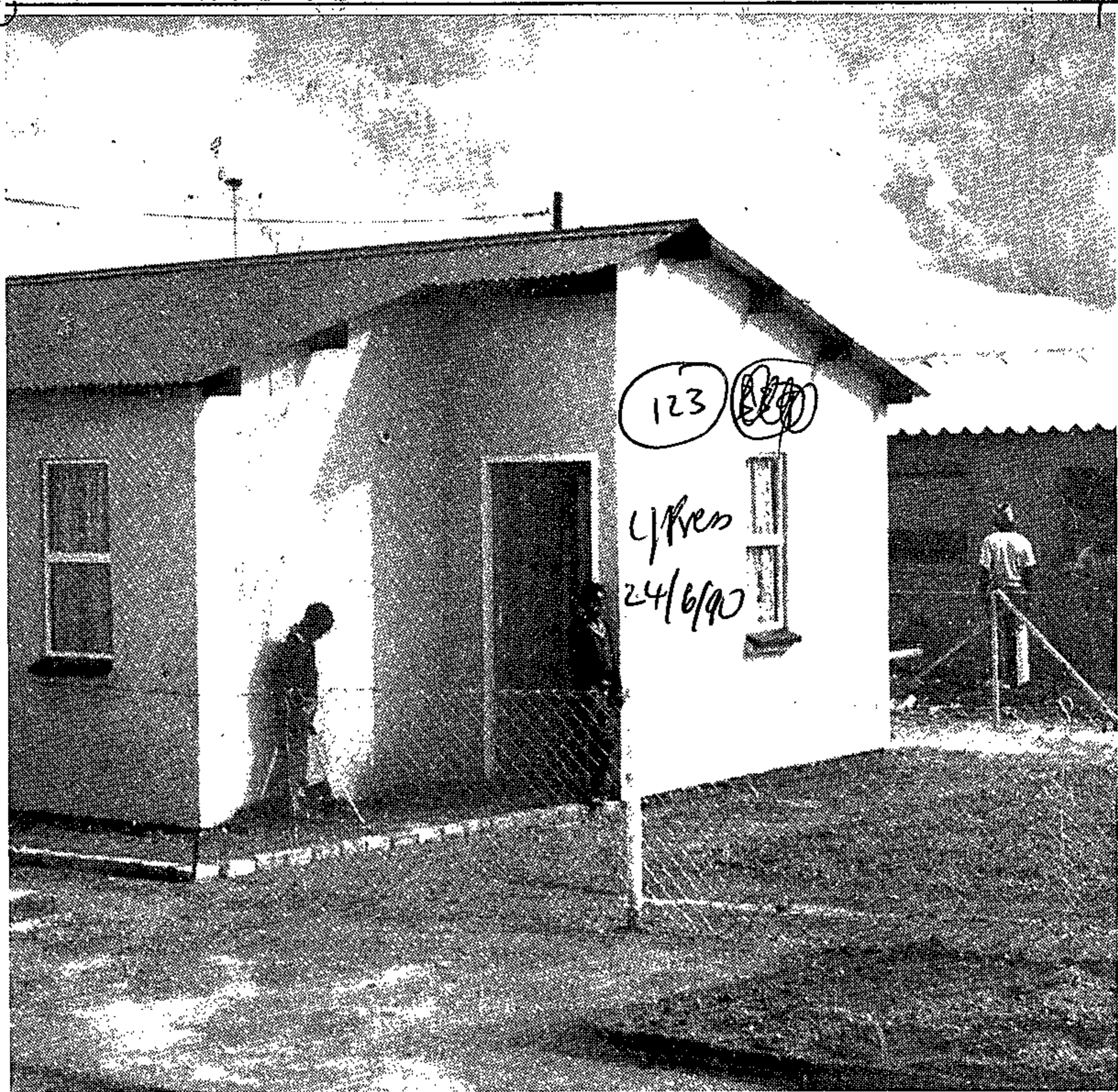
Some of the 150 low cost houses being built in Jouberton near Klerksdorp.
