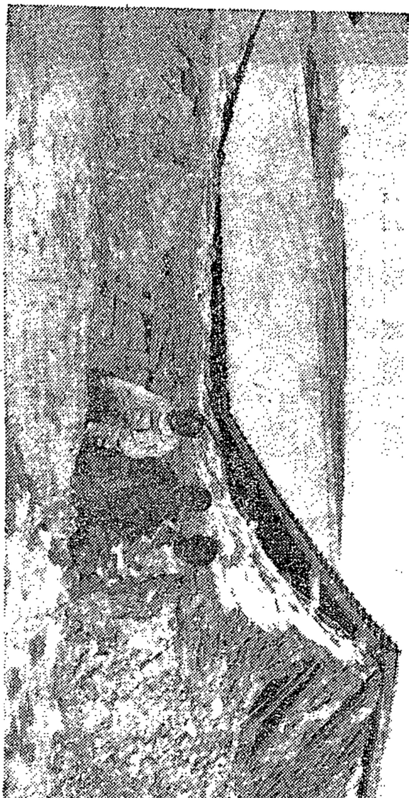
As the rain fell the foundations of this school subsided leaving 200 children with time on their hands and no school to attend
