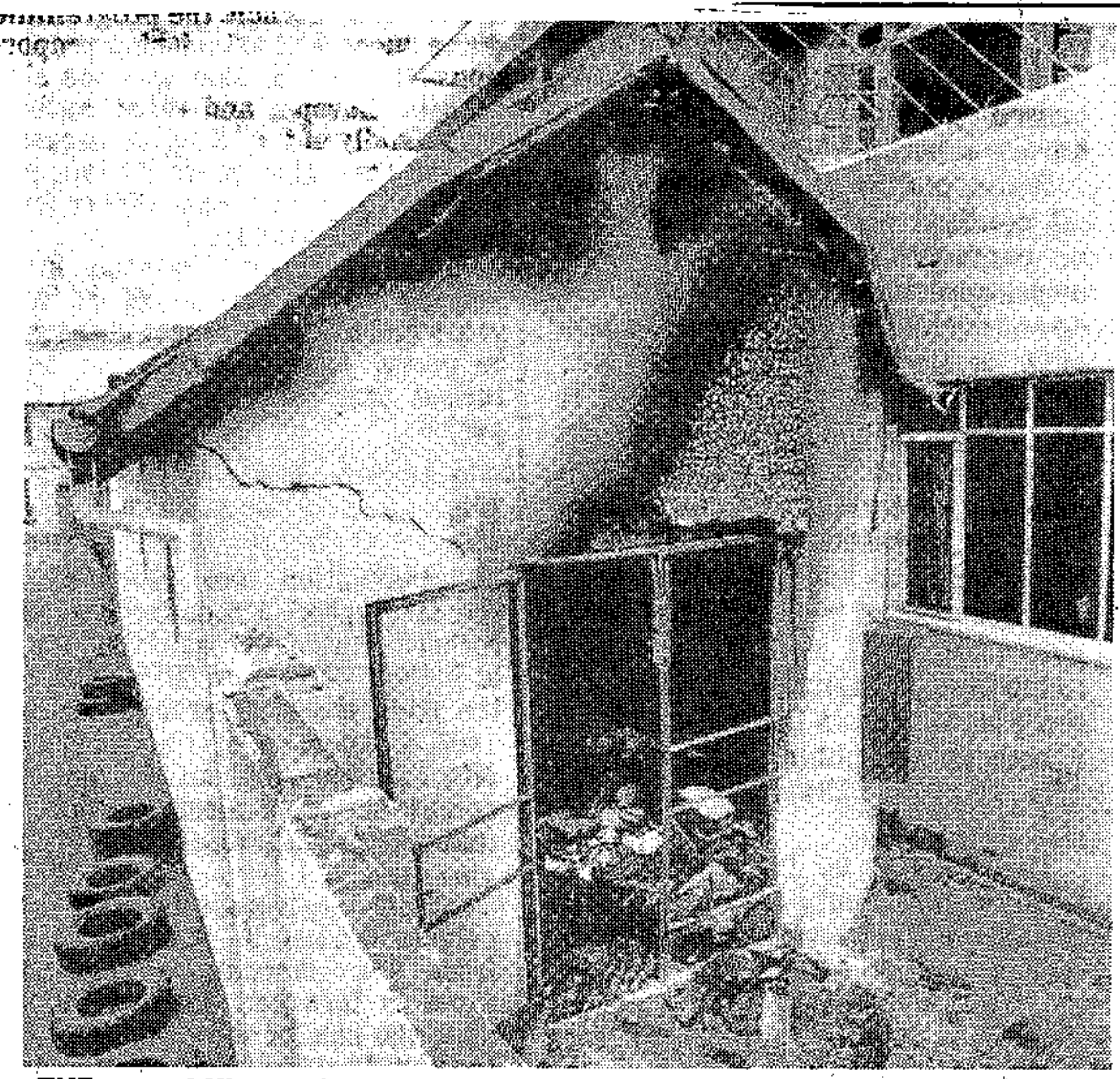
THE gutted Khanya House printing workshop — part of the headquarters of the Southern African Catholic Bishops' Conference in Pretoria — which was virtually destroyed when arsonists set the building alight with petrol and paraffin early yesterday morning.
