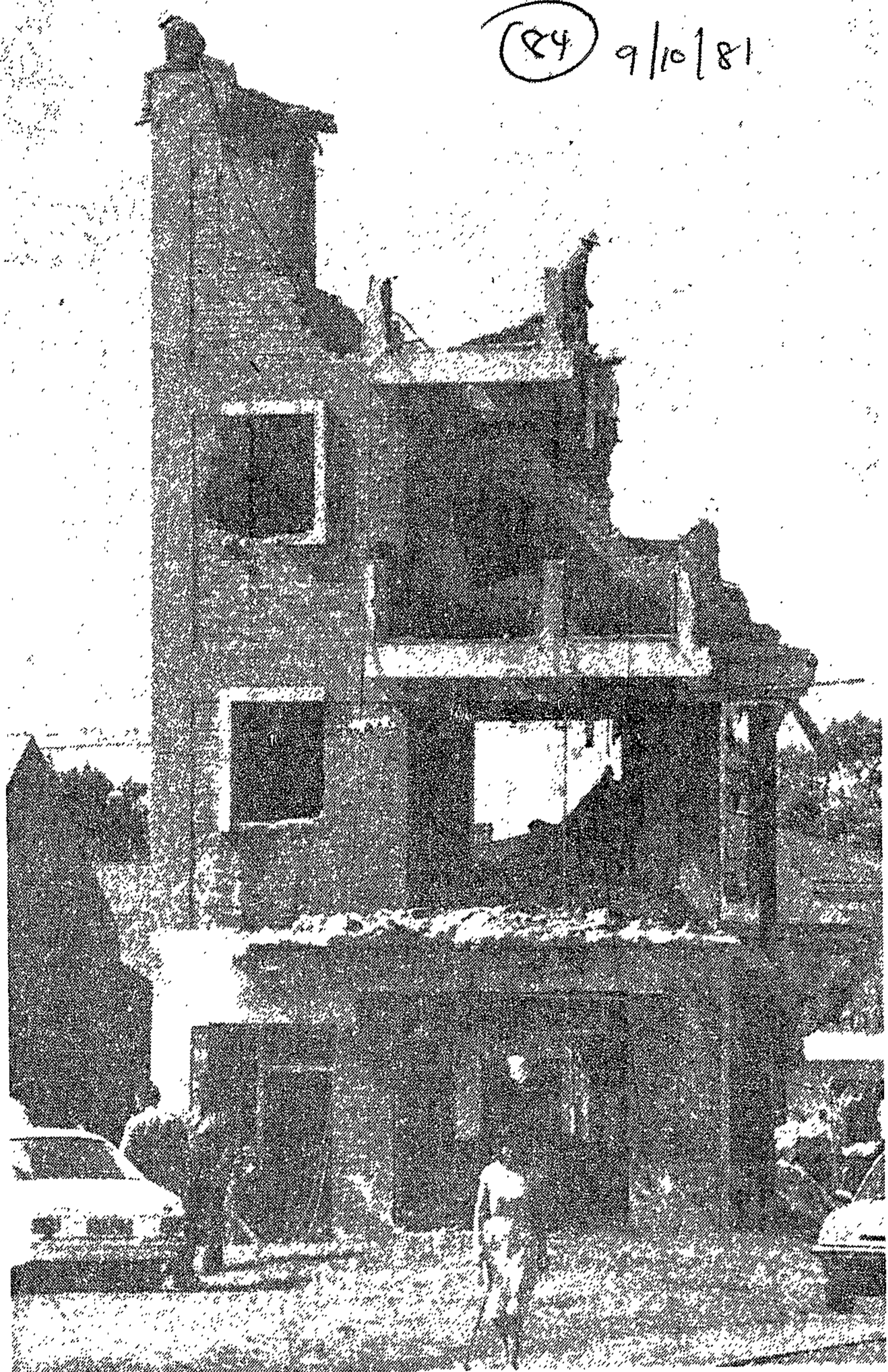
The demolition of this small block of flats in Pageview has been called "the deliberate destruction of a good building which had provided homes for several families." It will cost R250 000 to replace.
