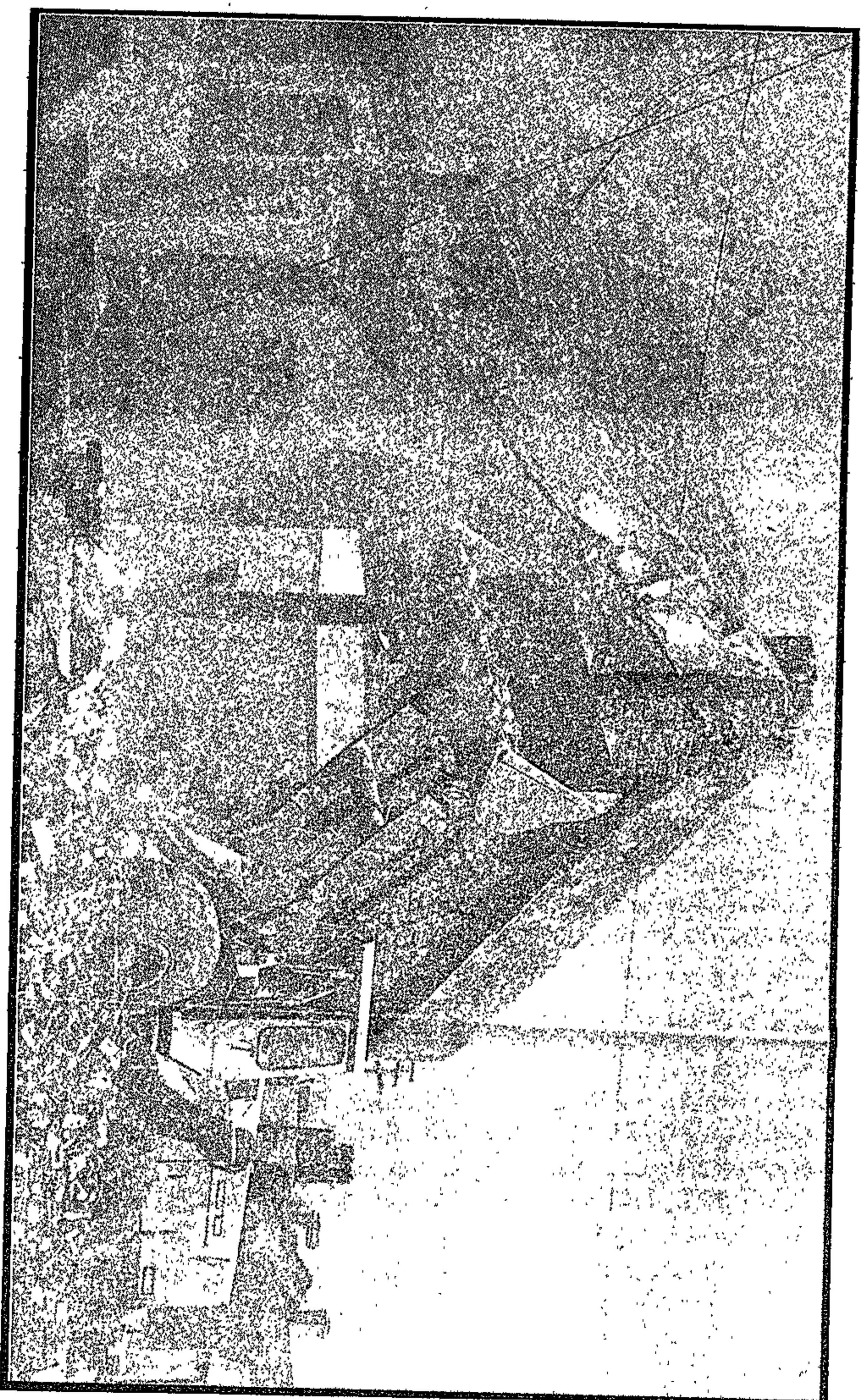
Clogging, choking dust as front-end loaders and bulldozers move in and old homes come tumbling down.
