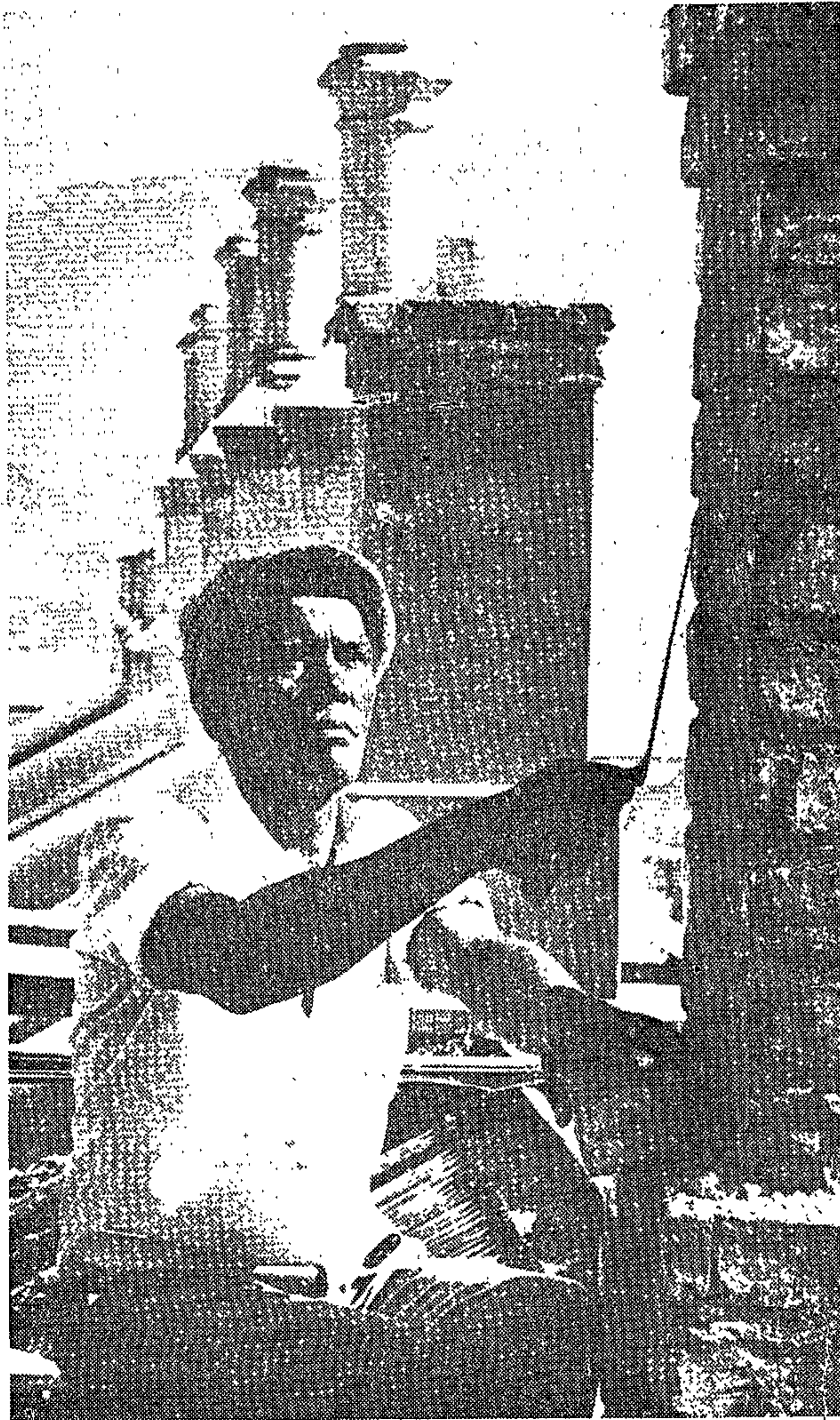
ABDULLAH HEWVEL replasters a chimney on one of the houses in Ashley Street, District Six, in preparation for its new white tenants.
