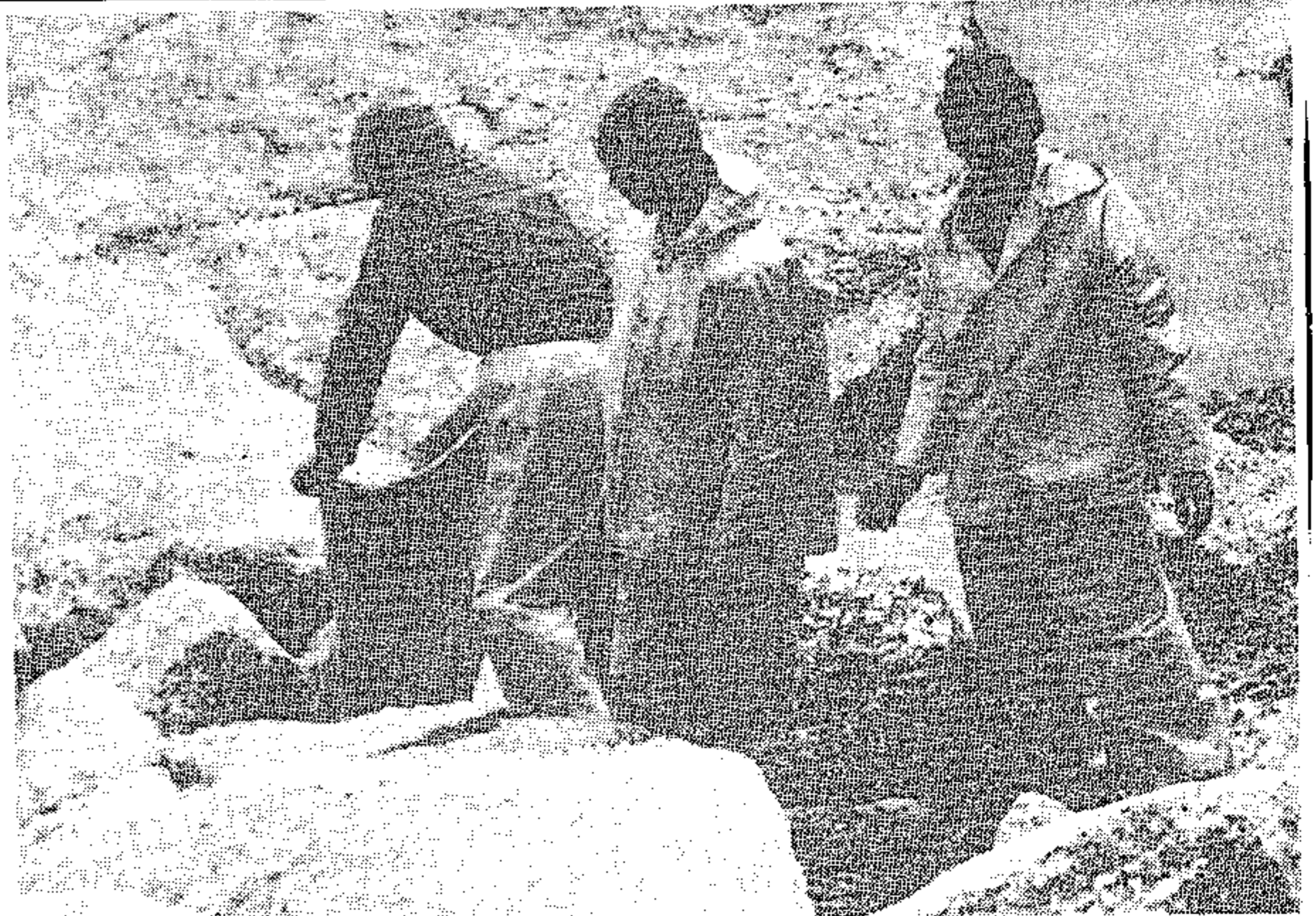
DUMPING SAND . . . Workers dump sand from an excavation site into the sea at Moses Beach, Clifton, yesterday. The city council has promised to take action to stop this.
