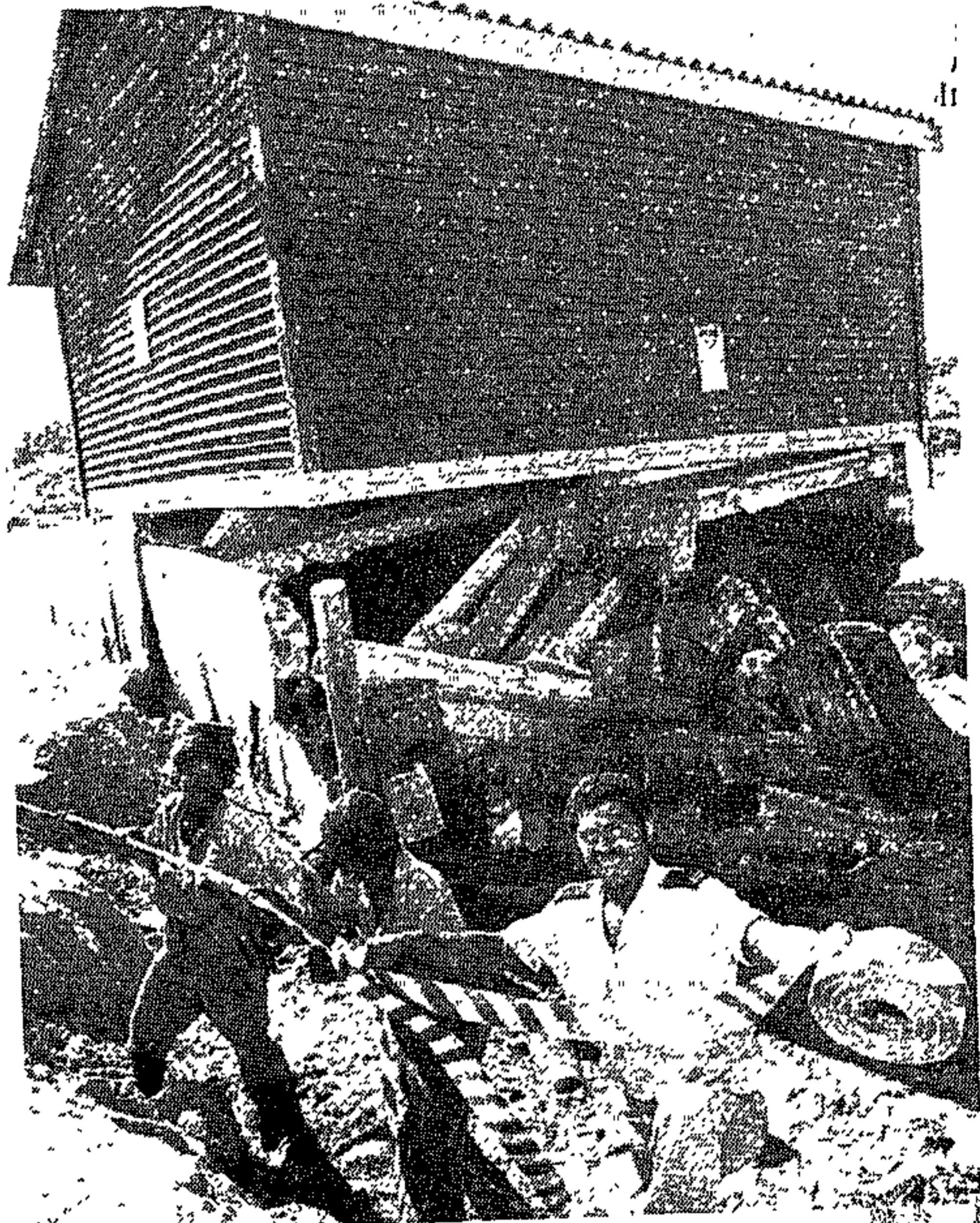
COLLAPSED: Council workers close access to a shop on Grotto Beach, Hermanus, damaged by floods.
