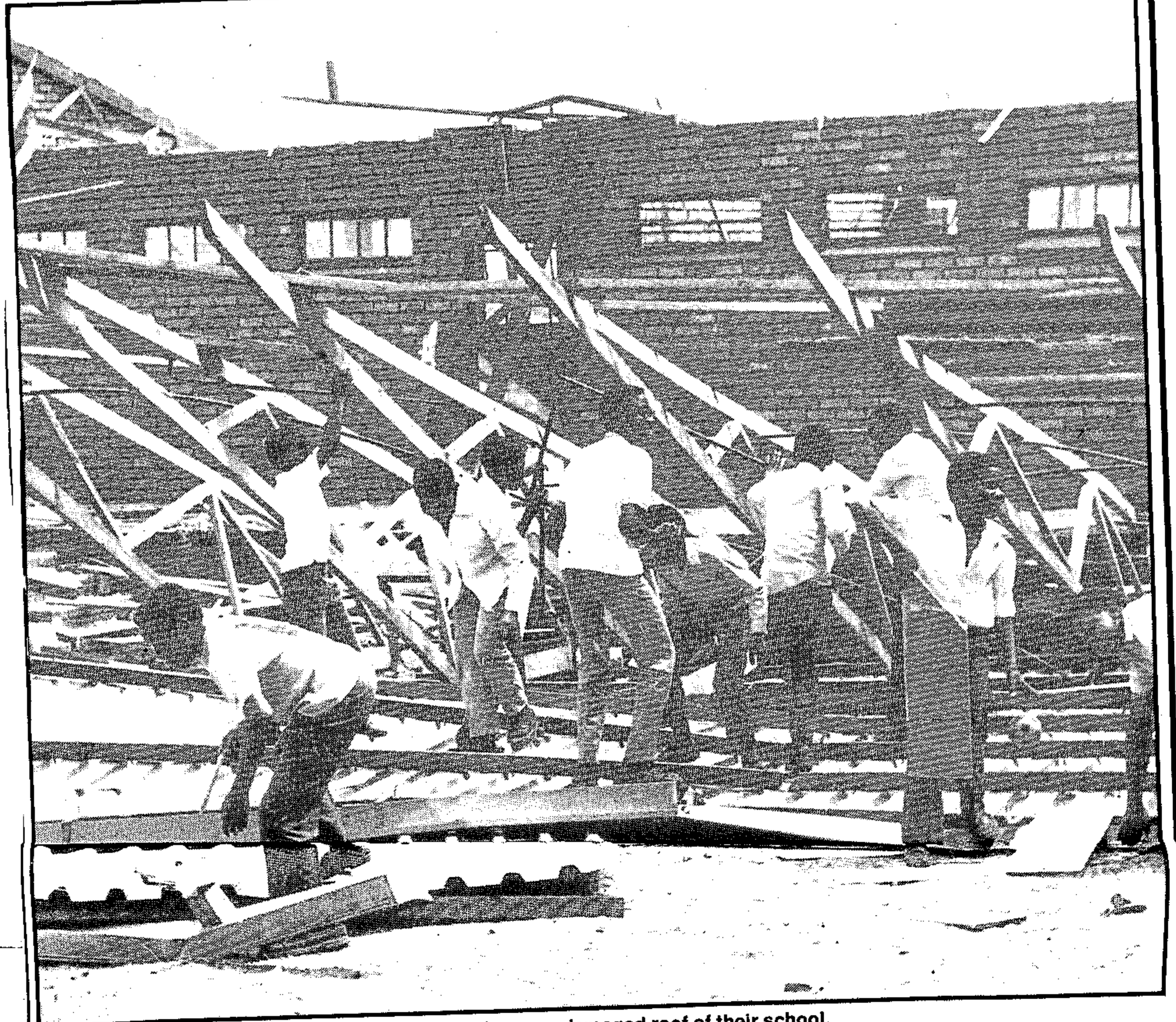
Pupils playing on a damaged roof of their school.
