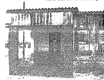
□ PRINCIPAL'S OFFICE: Dirty and mouldy walls near the office of principal Mrs Nomakhosi Mbane at Mkhanyiseli Primary School in Nyanga.
