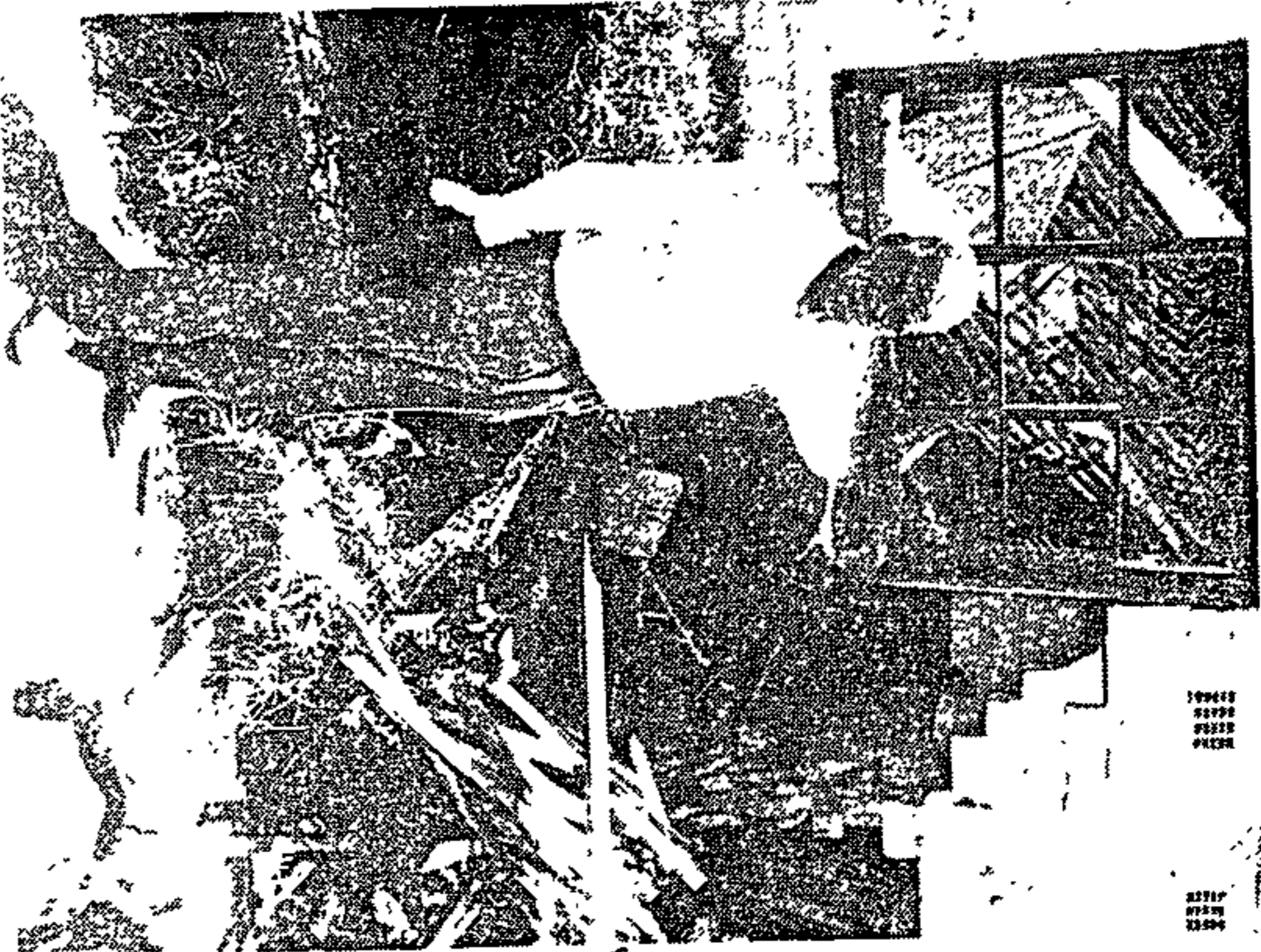
DAMAGE ... Mr Albert Lupizo points to the damage caused to his council home in Guguletu when a car smashed through the dining-room wall late on Friday night during Operation Thunderbolt. The driver had stolen the car in Diep River and became the subject of the chase when he jumped a red robot.
