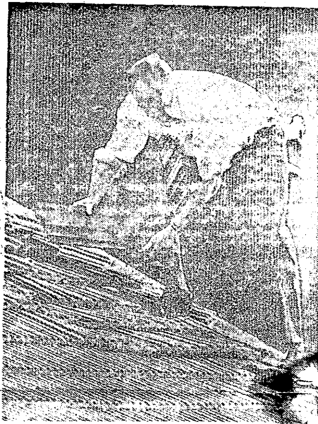
A plainclothes policeman removes tiles from the damaged roof of the servants' quarters to allow light to enter the room below.
