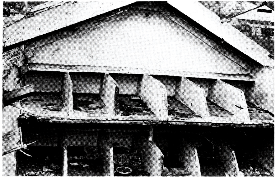
A compound dormitory in Crown Mines, during demolition, showing the concrete shelves or 'bunks' upon which workers had to sleep. Workers were housed in this compound until 1979. (Photo: Les Lawson)
