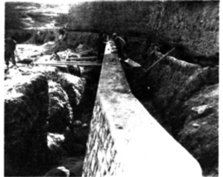
An example of mutual co-operation—American food forms part of the wages of these men working on an irrigation canal, a scheme under Morocco's national development programme.
