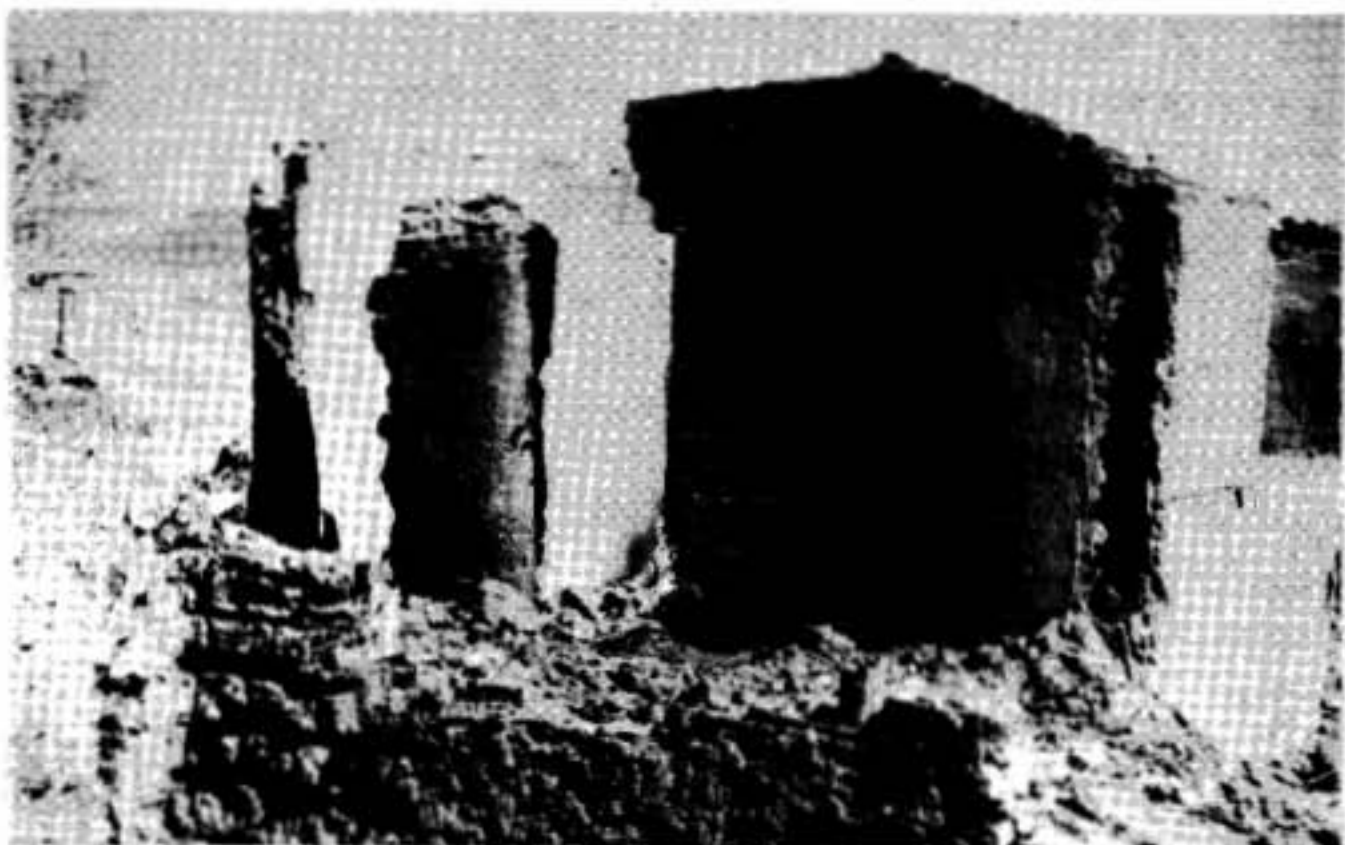
Damages at Ndundulu
