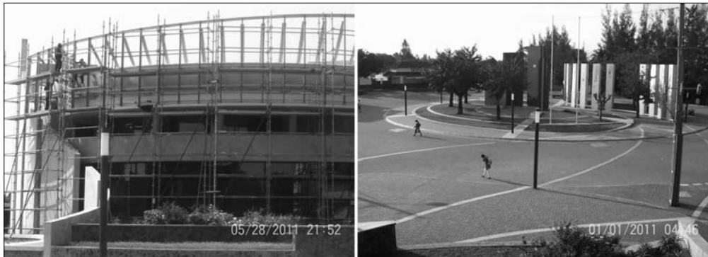
Figure 17.16a: Construction of the Interpretive Centre. Photo from the archives of the Matola Monument and Interpretation Centre
