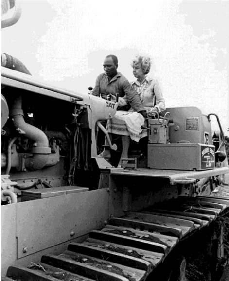
Fig 33. Part of the residential stock being demolished to clear the site for the Technikon. Mayor Sybil Hotz on the bulldozer at a ceremony on the site in the 1980s. (DUT archives)
